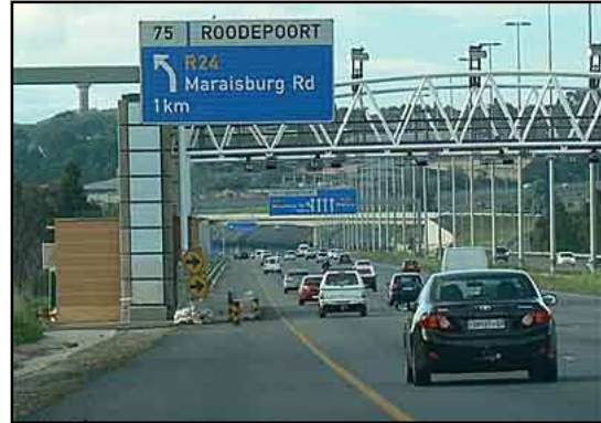
Overhead tag reading, automatic number plate recognition and vehicle classification equipment on gantry structure
